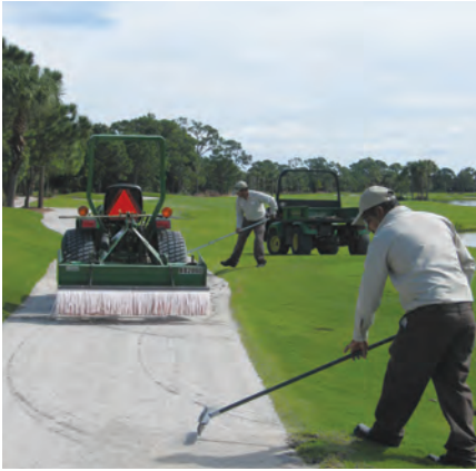
The Loxahatchee Club has pervious cart-paths made of concrete screenings. While they are considered a “low maintenance” item, they do require periodic maintenance and repair, especially after a very heavy rain.
