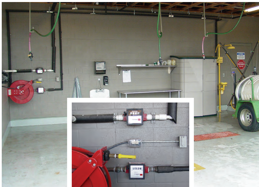
This is the main mix/load area. The concrete floor has a 36-mil chemical-resistant liner underneath and is sealed on top with chemical-resistant epoxy paint. The red grate covers the primary sump. A stainless steel mixing table, sink, eye wash and shower are some of the safety features. The recycled rinsate water is stored in a 500 gallon tank to the left. Photo by Larry Livingston, CGCS.
