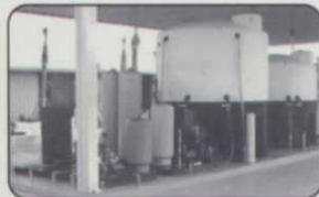
Wash Rack Systems – •closed loop •sewer discharge
