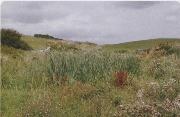
Establishment of a reed bed filtration system that cleans up waste water from a holiday park before it is re-used at Brighouse Bay Golf Club. This is also an excellent conservation initiative
