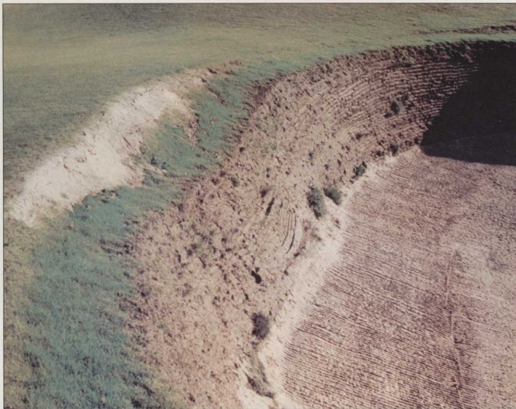
The collapsed face of Shell Bunker
