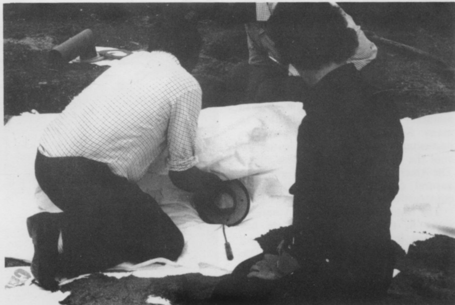
Outlet point being positioned in the PVC sheeting during the construction of the "Cellsystem".
