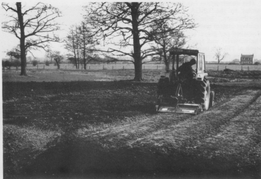
Rotary cultivation of the rootzone mix during the construction of the traditional green.
