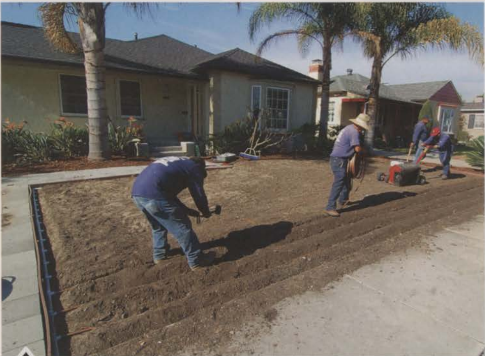
Two years ago, Garcia says no one knew about subsurface drip irrigation, but he now gets calls about it.
