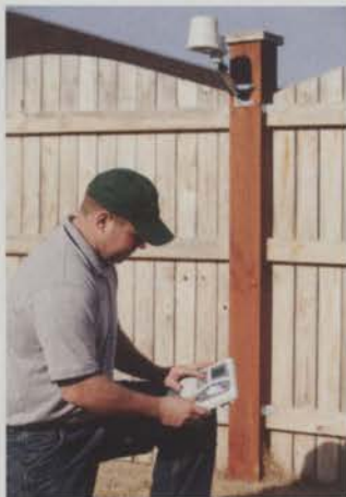
ET systems help save water.
