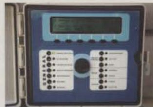
Contractors can't install smart technology and walk away.
