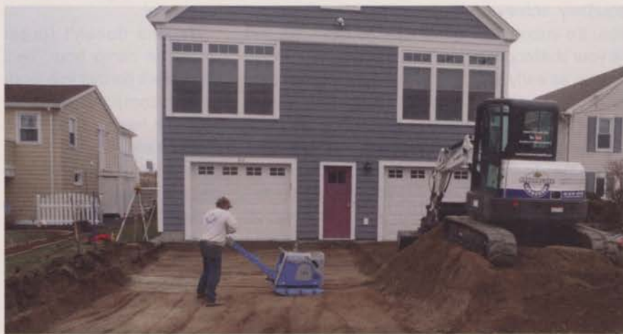
Sub-base and base compaction with the correct equipment will help insure quality installations on a job.
