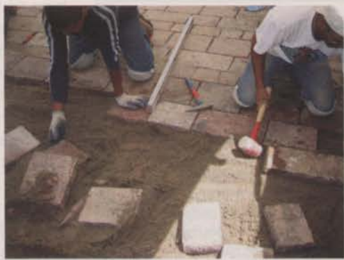
The subsurface of a permeable paver installation helps filter and mitigate rainfall.
