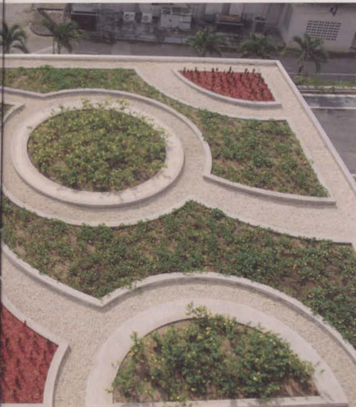
Aloha Landscaping and LMS Guam installed a green roof on the Coast 360 Federal Credit Union in Guam. The project was the first of its kind on the island.
