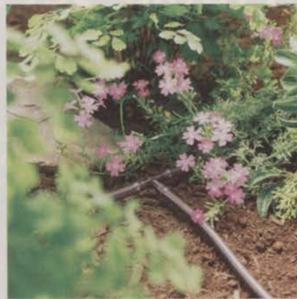
"Teas" like this one allow contractors to extend a drip line into out-of-the-way areas off of the main line. Photo: Orbit Irrigation
