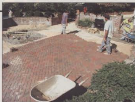
Paver installation requires a broad range of expertise that includes excavating, grading and compaction practices. Photo: Pine Hall Brick
