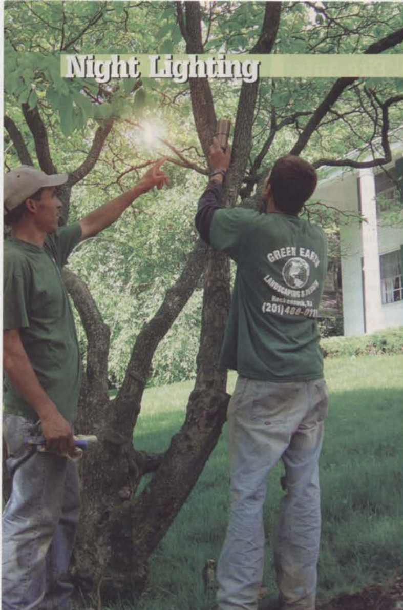
Creative placement of landscape lights in strategic areas help contractors showcase their work and increase sales. Photo: Green Earth
