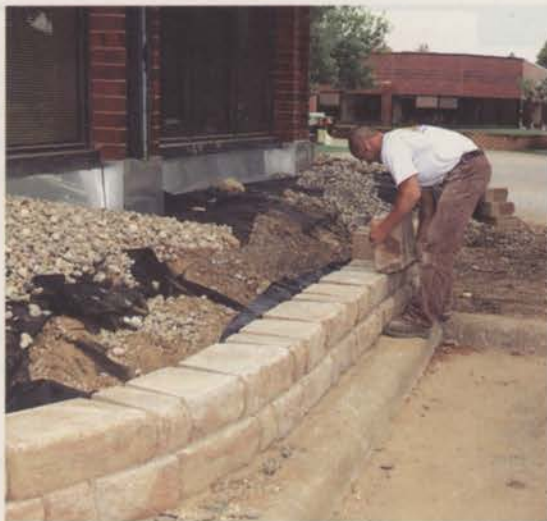
A retaining wall can add aesthetic appeal to a landscape while maximizing space. However, careful attention to detail and proper installation techniques are necessary for successful results. Photo: Anchor Wall Systems
