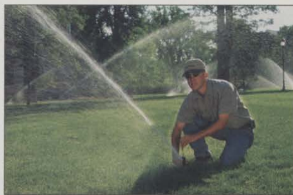
After installing an irrigation system, a tailor-made watering schedule is a must. Contractors should consider various factors when planning irrigation for a property. Photos: Hunter Industries (below), Rain Bird (above)
