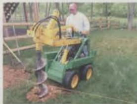
Compact utility loaders offer advantages in terms of site access, price, attachment capability and training. However, full-size skid steers can handle larger applications and offer greater lift heights and capacities. Top photo: Toro Sitework Systems, Bottom photo: Kanga.
