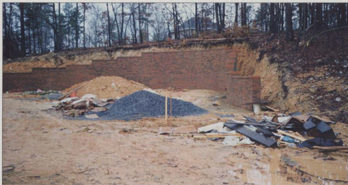
Access issues and steep slopes create installation obstacles. Photo: Watters & Associates Landscape
