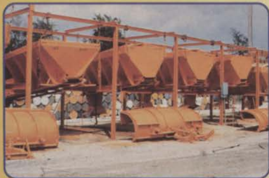
Spreader chains and interior of spreader boxes, tailgate or V-bottom, rust and corrode during off season storage.
