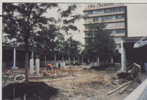
Equipment access into the Old Orchard open-air shopping mall was difficult for Church Landscape employees, particularly after building canopies were installed. Photo: Church Landscape
