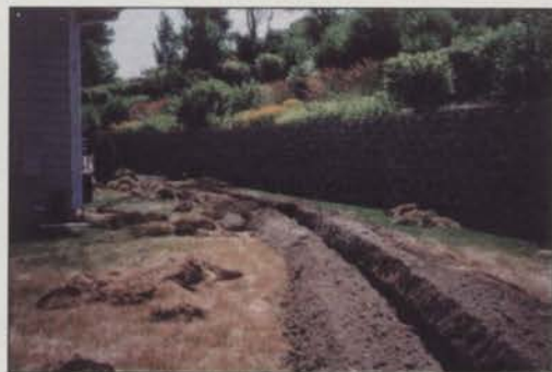
To control a severe drainage problem on one site, Perficut employees had to dig a trench along the back of a condominium complex partly by hand to lay piping and draining tile. Photo: Perficut
