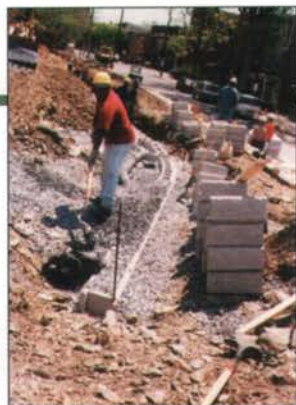
A crew works on installing a segmental retaining wall. Photo: Allan Block Corp.
