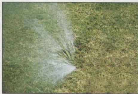
Pressure problems can undermine the effectiveness of an irrigation system. Here, pop-up spray heads work ineffectively in a low pressure situation.
