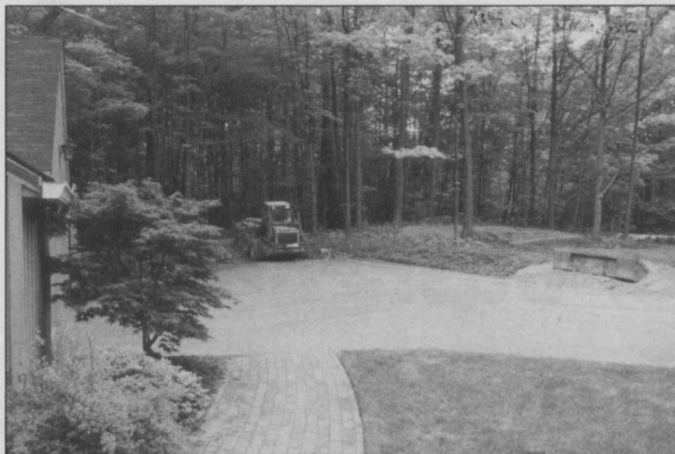
The first step in the demolition process was the removal of the dead, half-dead or rotten trees. Also removed were the trees and ornamentals that were in the area where the lawn was going to be added. Photo: The Pattie Group
