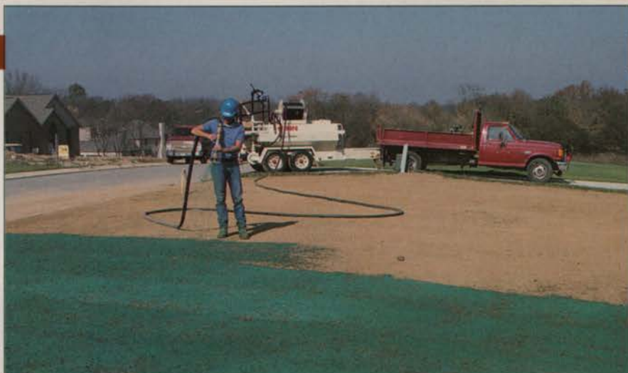
Although hydroseeding will usually require higher capital expenditures, many contractors appreciate the fact that it is a task that can be performed with minimal labor. Photo: Finn
