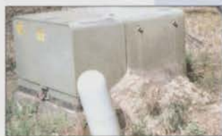
Fire ants may colonize near high voltage areas and cause damage.
