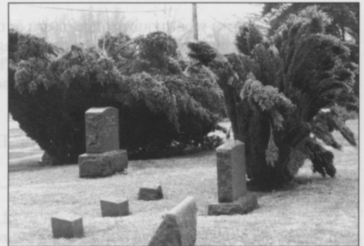
Bushy ornamental plants show damage from the weight of heavy snow and ice. Credit: Davey Tree
