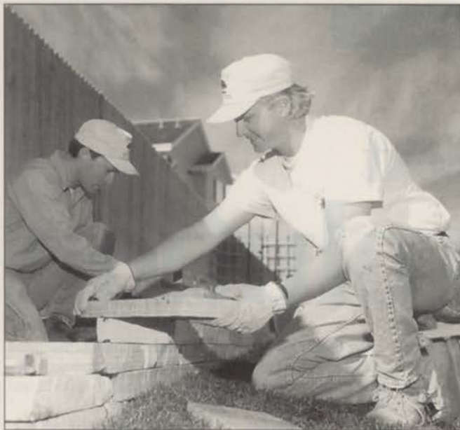
Landscape design and installation have grown into a major part of Swingle's service mix.
