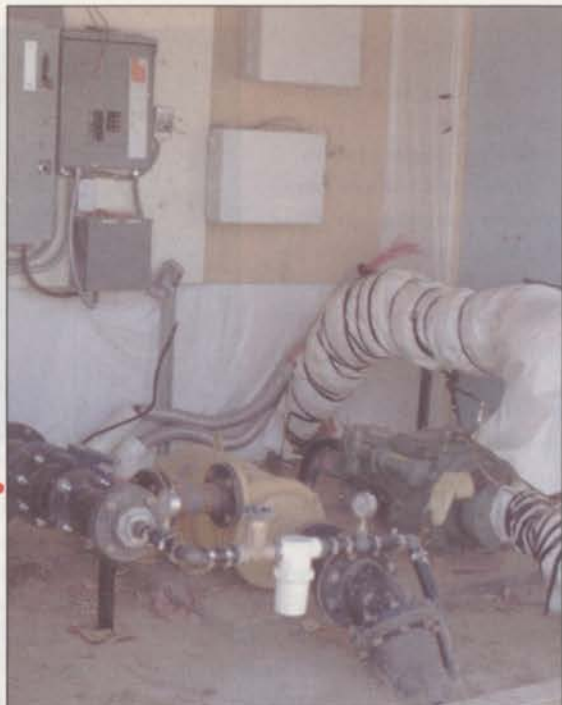
Actual installation conditions play a major role in the ability of pump system components to provide adequate performance.
