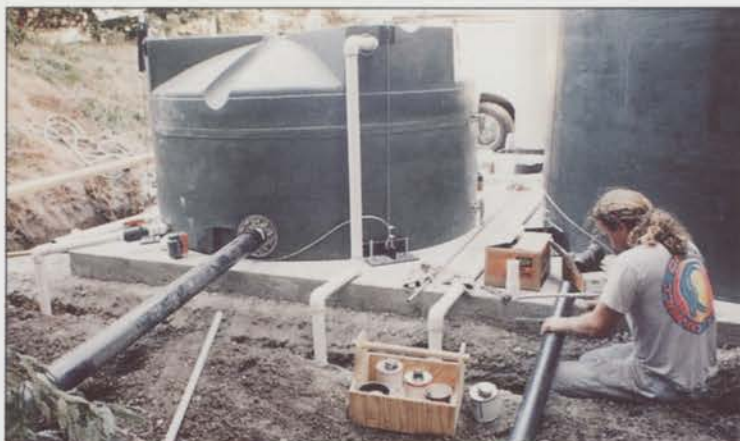
Graywater systems aren't particularly difficult to build or maintain.
