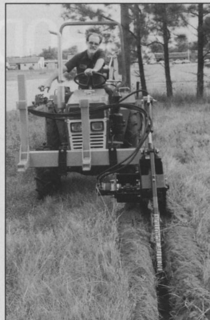
Ongoing education is needed to promote the benefits of automatic irrigation systems beginning with the initial installation.
