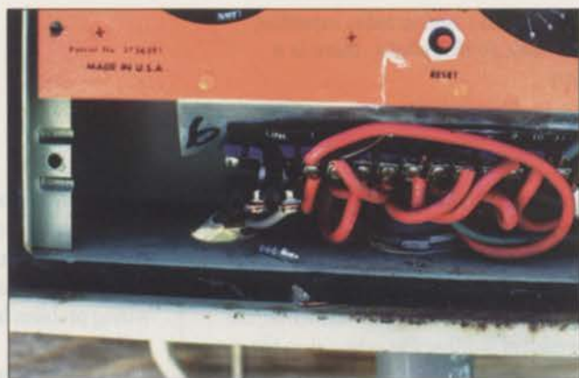
An electrician should periodically check the control panel. At left is a defective terminal strip at 110-volt connection.
