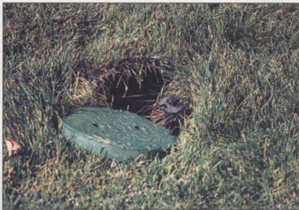
When a valve is installed too high in the turf, the lid won't properly fit the system. Photo: Larry Keesen
