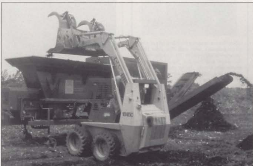
A front-end loader and a tub grinder are staples of composting.
