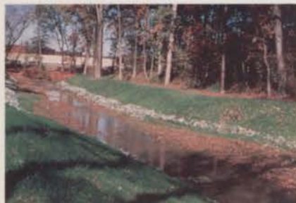
The banks of Stewart Creek after grass had grown up through the Enkamat matting.
