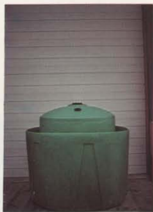
Bulk storage tank within a diking system.
