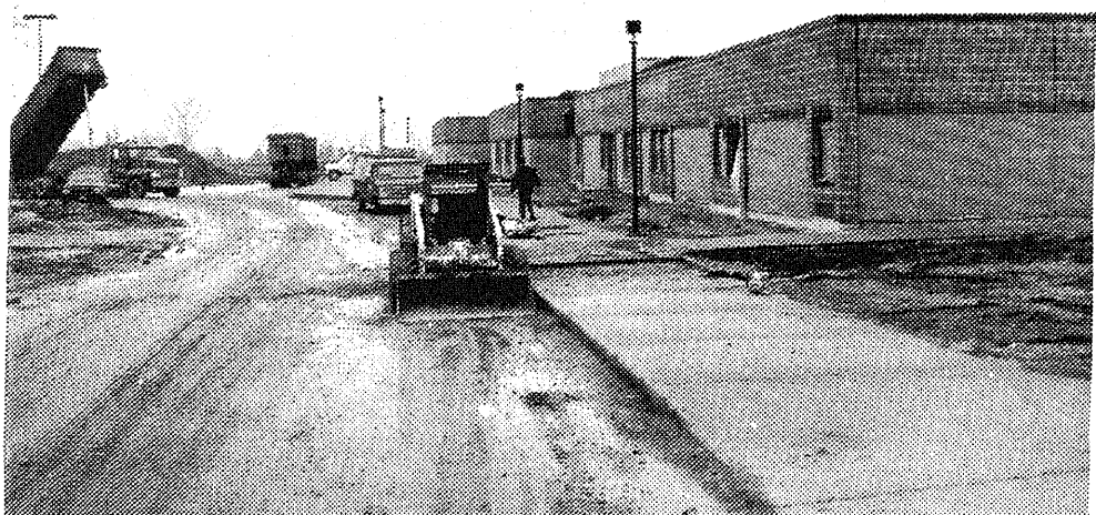
The new USA Middle School looked far different back in February, when these muddy pictures were snapped. Exterior work had been completed, but much interior work had to be done, before students could begin their 1995-96 school year in the new $5.7 million complex adjacent to USA High School.
