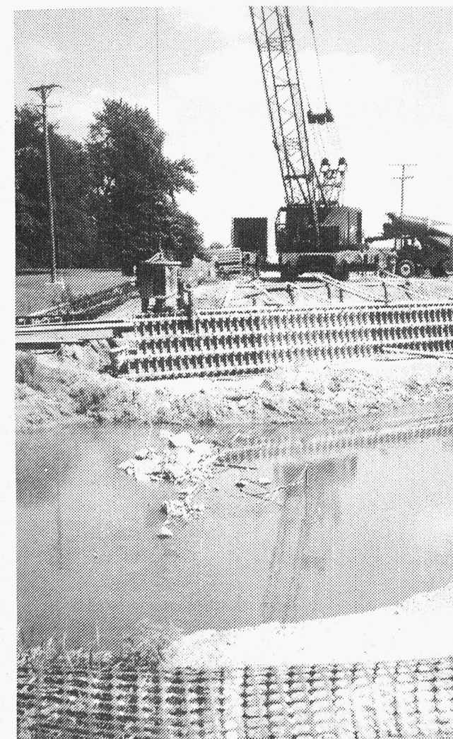
A BRIDGE TOO FAR: Don't try to cross the Filion Road bridge over the Pigeon River just south of Hayes in the near future, as this photo shows. The new structure being built by the Huron County Road Commission replaces the hump-back bridge there. Completion is expected this fall.
