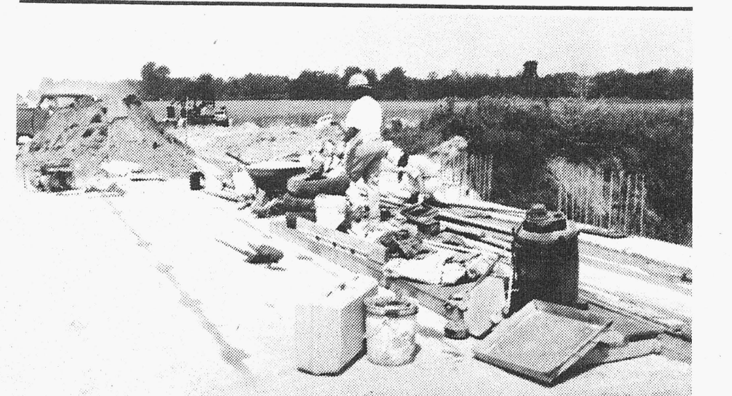
DESPITE 90-PLUS degree temperatures and lots of rain, work continues on the replacement of the Geiger Road Bridge just off M-25 near Bay Port. Here, two of McDowell Construction's employees were busy doing cement work between storms last week. The bridge is between M-25 and Kuhl Roads. It has a $152,000 price tag, and McDowell Construction of Columbiaville is doing the work. MARY DRIER PHOTO
