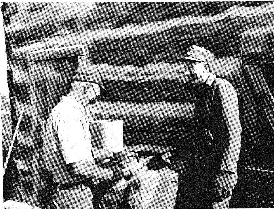
CHIMNEY WORK: Elkton's Log Cabin is getting a new addition as members of the Elkton Historical Society construct a fieldstone chimney for the cabin. The stones were donated by Earl Buschlen, from an old barn on his property south of Elkton. Here, Vern Powell, left and Milton Young work on the chimney which is rising at the rate of about a foot a day. The finished chimney will stand about 22 ft., Powell says, and will be a working chimney. AMY HEIDEN PHOTO
