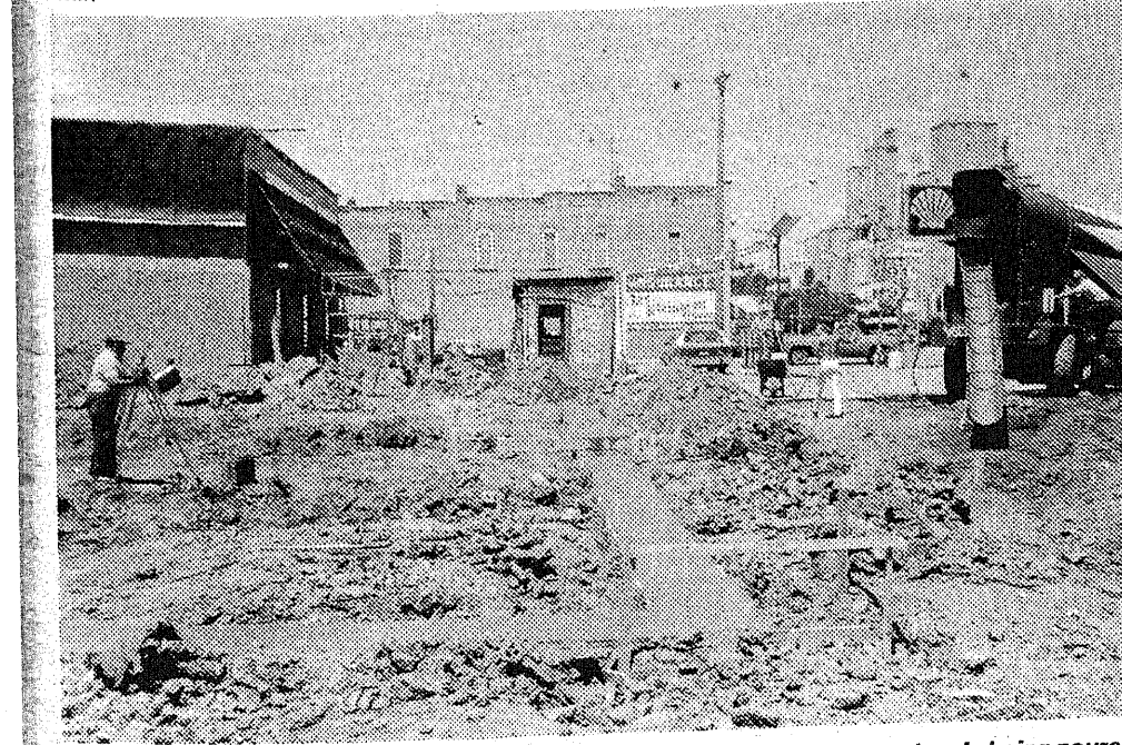
FAST WORK: The footer for a new building at People's Oil & Gas was already being poured last week at the site of the house that was just moved down Main Street days before. The structure will house a new convenience store, which will join a laundromat currently under construction in what was formerly part of the service area of the business. RICH SWARTZENDRUBER
