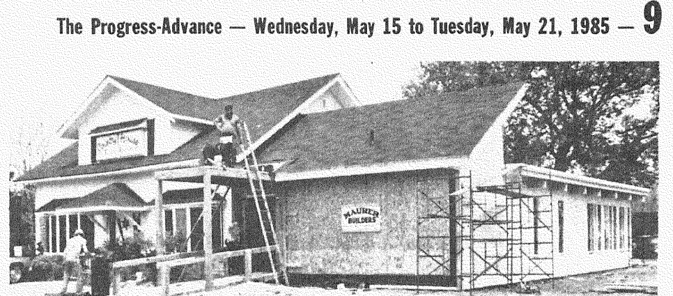
CASEVILLE MODERNIZATION: A building program at the Country House restaurant Caseville, should be completed within the next three weeks, according to owner John Parr. The modernization on the south side of the historic building at 6567 Main Street will be barrier free and will have bathrooms on the main floor. A skylight will provide natural lighting and a co-fee shop area will be created in the present building. No additional seating is anticipated, Parr says, and business goes on as usual around the construction. RICH SWARTZENDRUBER PHOTO
