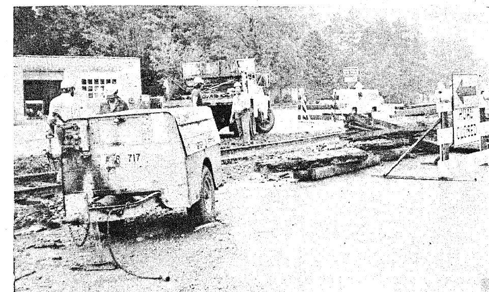
HIGHWAY CLOSED: Use of M-142 (Pigeon Road) just west of Pigeon was stopped all day Monday and part of Tuesday, as a Chesapeake and Ohio Railway "Crossing Crew" removed decaying rail ties at the crossing and replaced them.
