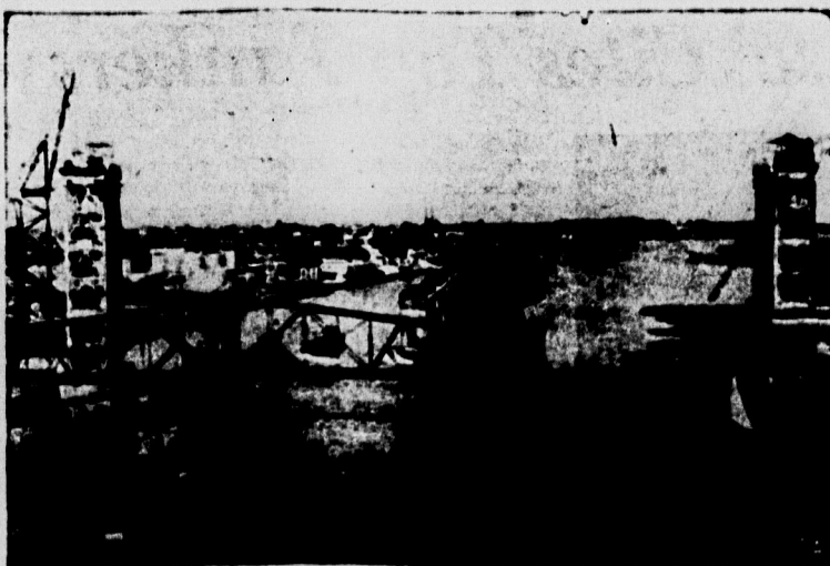
CENTER OF WORLD'S longest vertical lift bridge is floated into place in Arthur Kill, New York, Sunday, behind old span it replaces. The bridges connect Elizabethport, N.J., and New York City's borough of Staten Island, Baltimore & Ohio trains will be using the new span by July 15.
