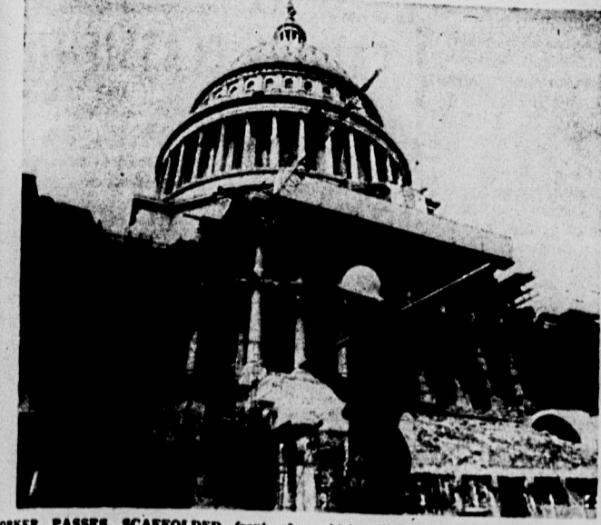
WORKER PASSES SCAFFOLDED front of Capitol building during renovation work which will extend east front of historic structure.
