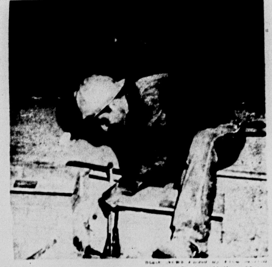
A workman drills on the fourth floor of Berkeley Hall as 50 new offices are being put in. The continuous noise of the workmen have forced many classes to be let out early.
