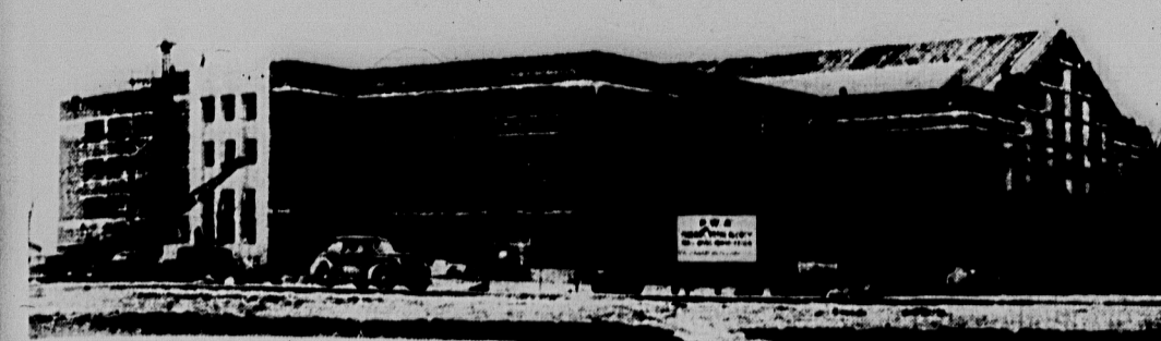
Although Jenison fieldhouse in general is far from completion... the fieldhouse proper which occupies the western part of the building is far enough advanced to permit the playing of the State-Tennessee Basketball game there Saturday night.
