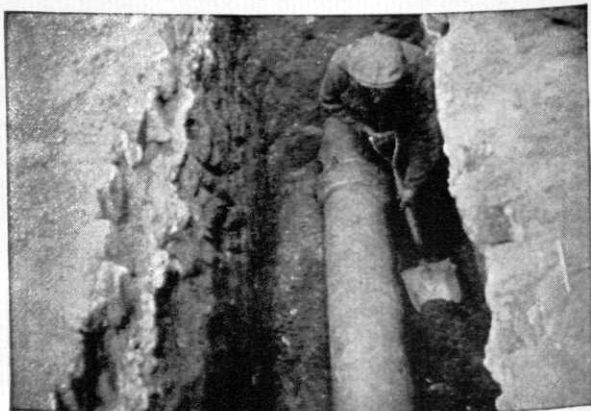
Section of 130-year-old cast iron water main still in service in Philadelphia, Pa.
