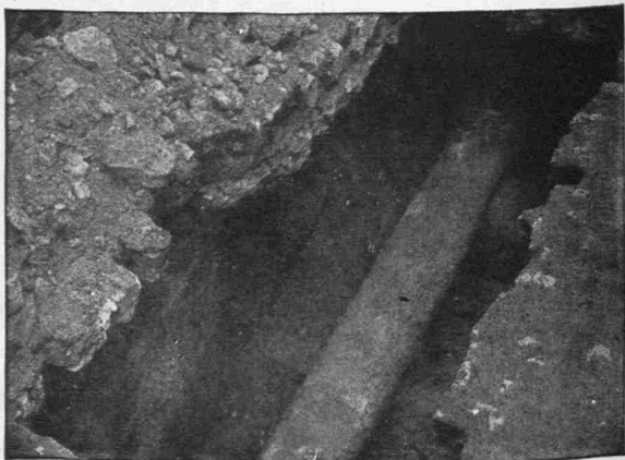
Section of 114-year-old cast iron gas main still in service in Baltimore, Md.
