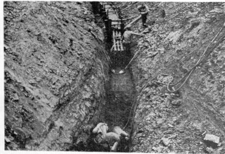
CONDUIT TRENCH BEING CONSTRUCTED AT THE GRAND RIVER CROSSING OF JOHN C. LODGE EXPRESSWAY
