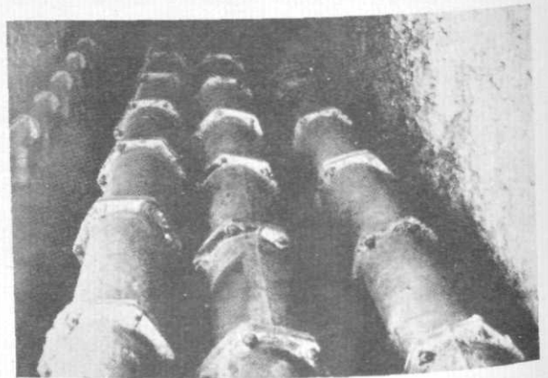
Section of 285-year-old cast iron water main still serving the town and fountains of Versailles. France.
