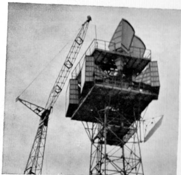
Microwave relay towers assure reliable land transmission of telephone, radio, television and data traffic—with complete flexibility.
