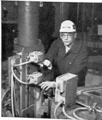
FRANK PERETIN, E.E., PITT '60 —As an engineer in the Johnstown, Pa., Plant Electrical Department, Frank's duties involve power generation and distribution, drive systems, and electronic controls.
